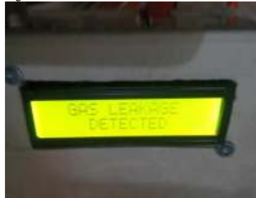
Fig.11: LPG detector system with gas concentration greater than set reference.
