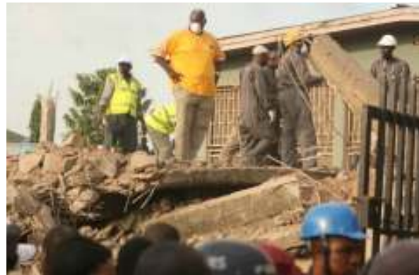
Picture of a 3 storey building belonging to Foursquare Gospel Church that collapsed in Ojodu-Berger Area of Lagos on May 8 th , 2013. Several construction workers were trapped in the building
